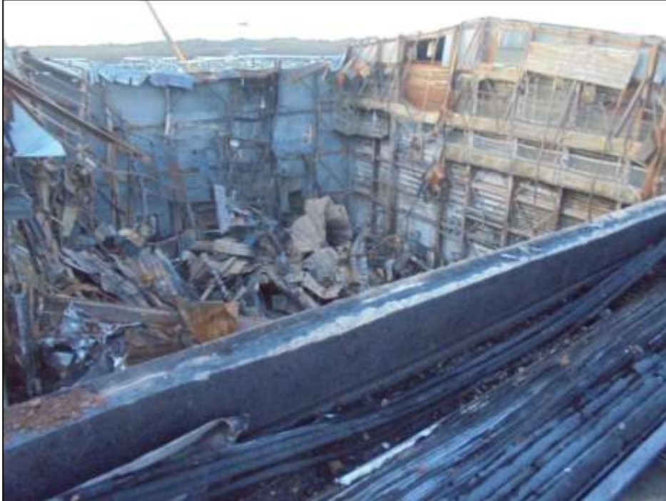
Figure 2 Fire Damage to Main Building
