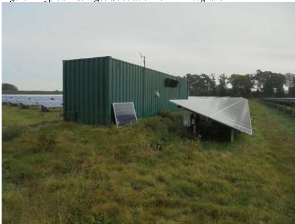
Figure 1 Typical Packaged Substation for PV Integration
