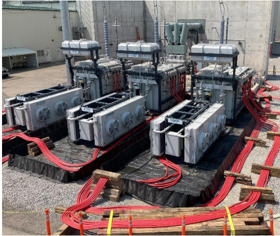
Assembled single phase multi ratio resilience GSU transformers 250 MVA (Voltage range: HV 115-400kV, LV 12-34,5kV) (photo: Siemens Energy)
