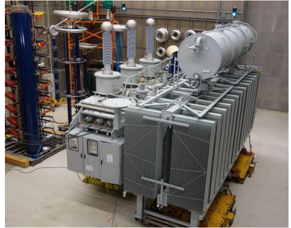
Compact area station transformers Type 2: Synthetic ester liquid Midel® 7131 (photo: Siemens Energy)
