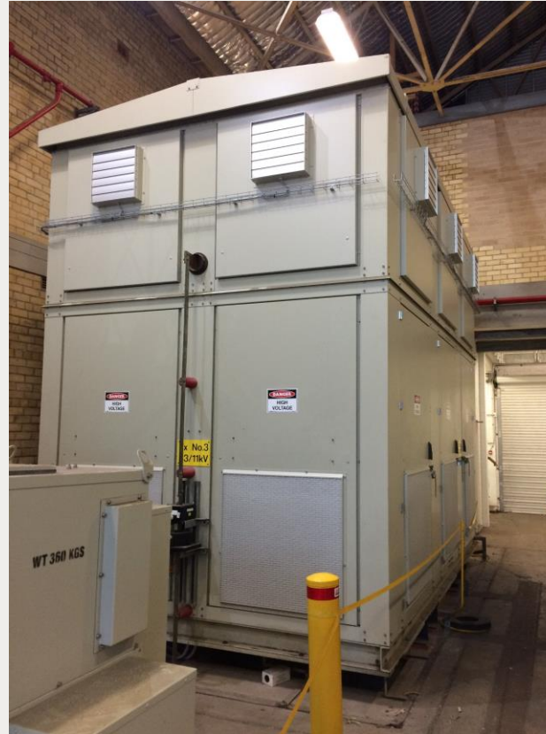
Sealed enclosure – fans & filters
