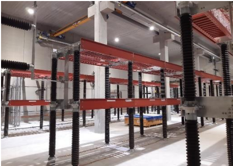
Fig. 4: Picture of the rectifier hall in Supergrid Institute High Power Laboratory
