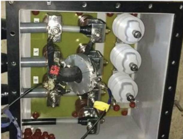
Figure 3 - PD Sensor installed
