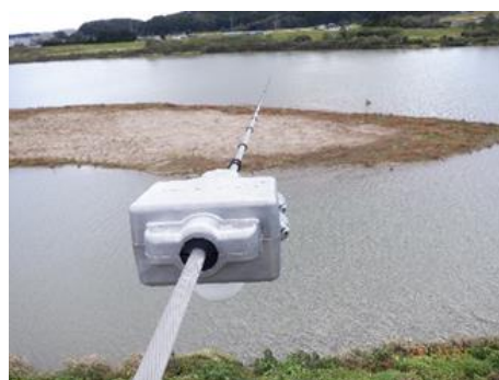
Fig.1 Ampacimon sensor installed on the target span
