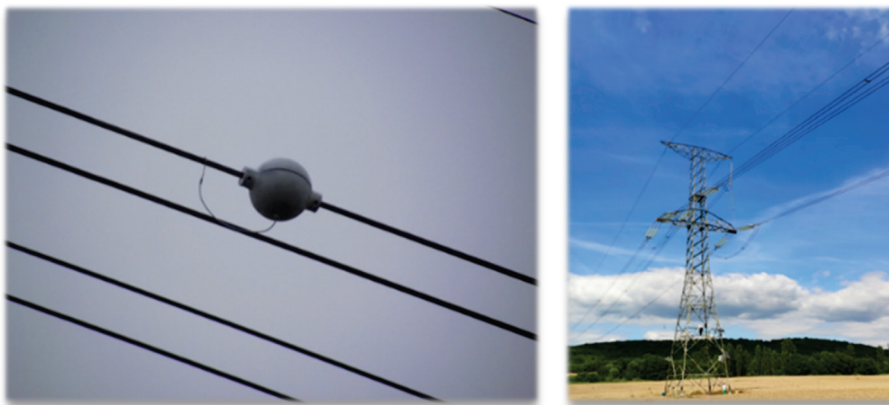
Figure 3. Low-cost sensor under field test on a 400 kV power line
