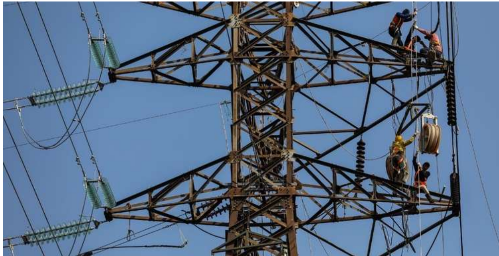
Fig.3 Replacement of ACSR410 mm 2 single conductor to ACFR mm 2 2 conductor (left line is ACFR with tensioned work completed)
