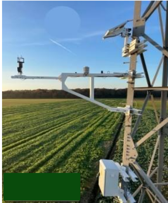
Figure 2: weather station fixed on a structure
