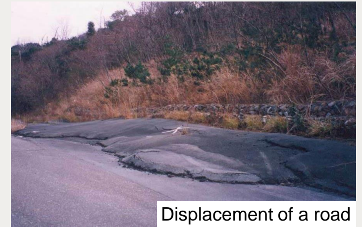
Crack on a road
