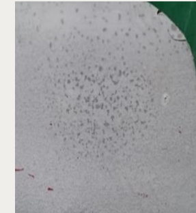
Poor quality <Coating peeled>
