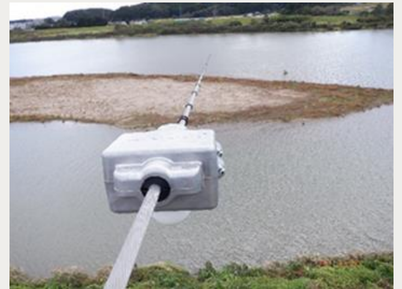
Ampacimon sensor installed on the target span
