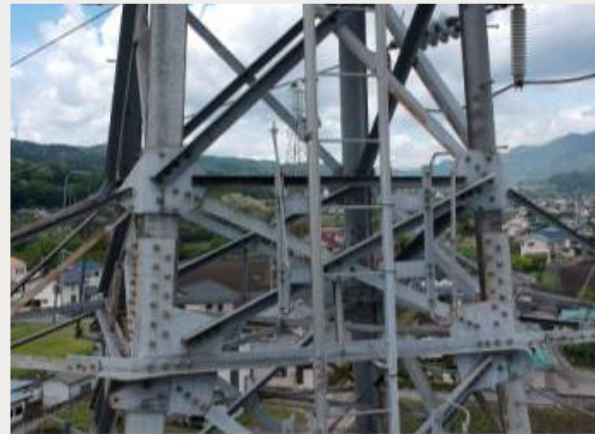
Overhead view of the steel tower containing the rusted area
