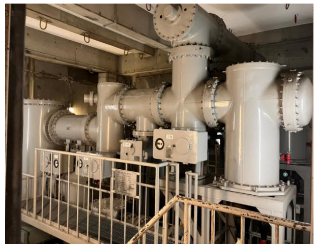
Figure 5: Example of a narrow GIS substation.
