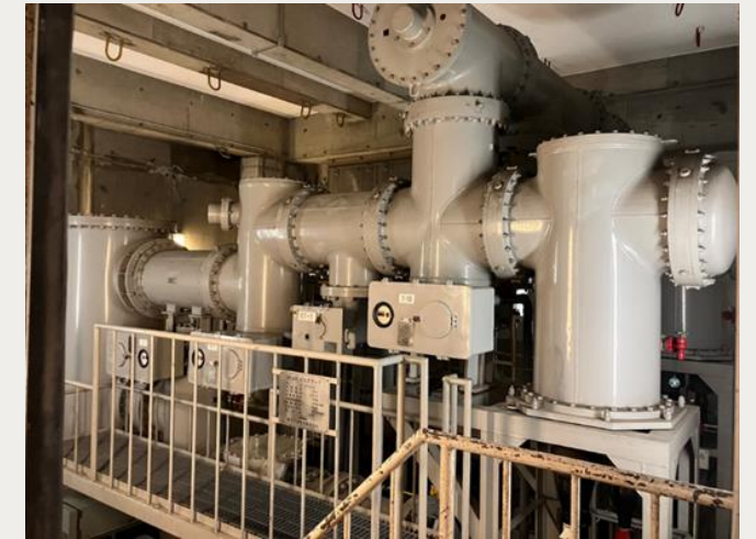
Example of a narrow GIS substation
