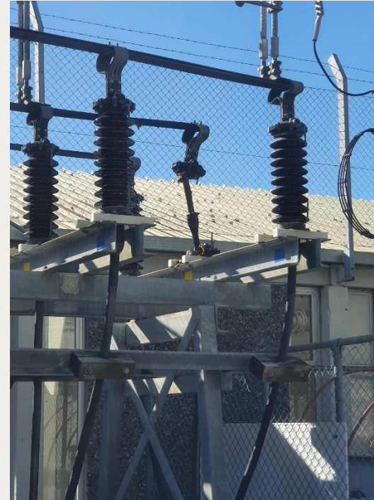
GFD Cable Sealing End Failure – sending in staff to inspect similar remaining in-service assets for damage
