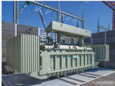
250 Mvar VSR, 440 kV, acceleration sensor on tap-changer head cover
