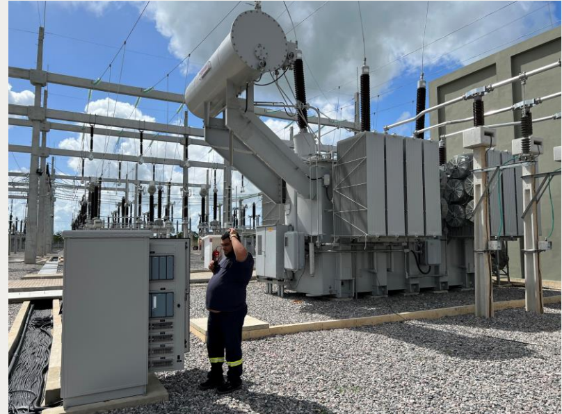
Commissioning in DSS Mata Norte
