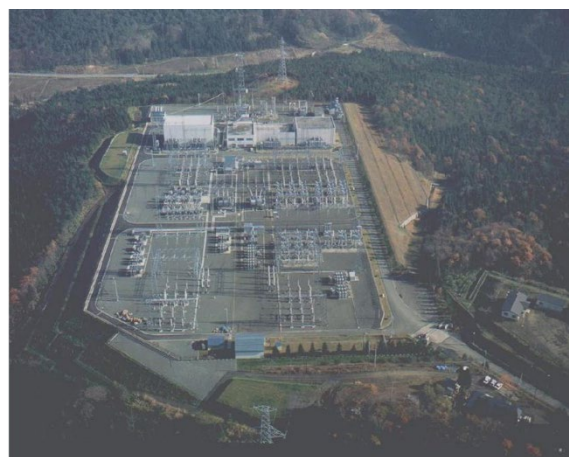
Kamikita converter station
