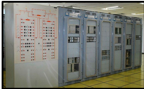
Figure 1a) Control System panels at Rectifier Station
