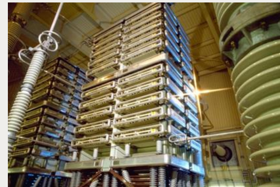
Thyristor valve tower (Pole 1 of Hakodate C/S)
