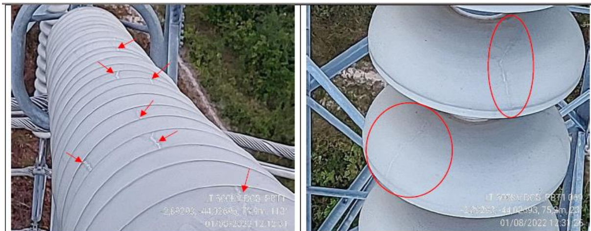
Figure 6 – Atmospheric Discharge Identification – Tower nº 69
