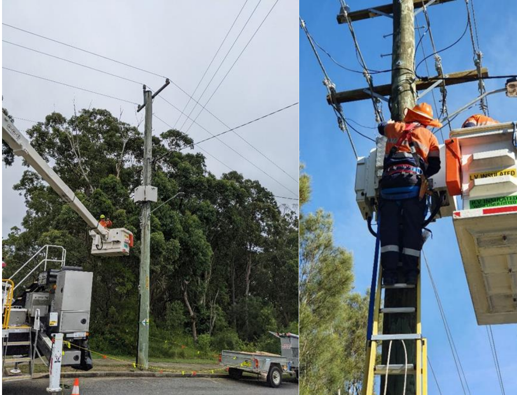
Figure 2: A typical installation of a three-phase LV STATCOM
