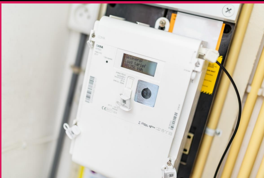
Seasonal voltage measurements at LV feeder ends
