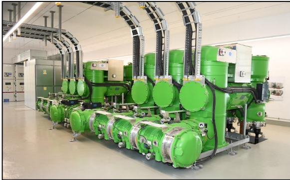
Figure 6: C4-FN mixture GIS, 6 bays of single busbar configuration in the substation Zernez (CH)
