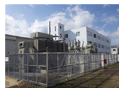
Fig. 5 Appearance during energization test of 2 Units of three-phase, 10 MVA-66 kV transformer
