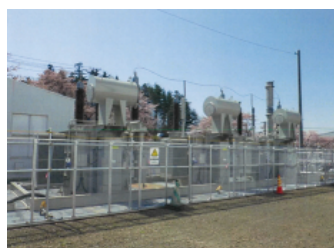
Fig. 6 Appearance during long-term energization test of 3 Units of single-phase, 2 MVA-154 kV model transformer
