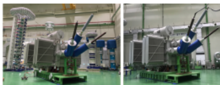
(a) Dielectric test (b) Temperature rising test Fig. 5 Type test of transformer for modular substation
