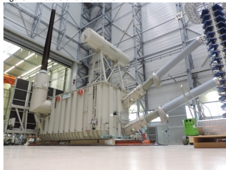
Figure 2: Picture of transformer:
