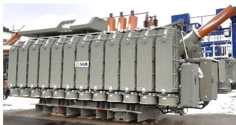
Figure 1. Photograph of the completed 80 MVA unit filled with NYTRO BIO 300X.
