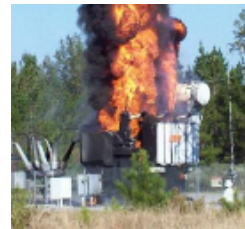
Figure 2: Bubble formation as a possible cause for transformer failure? Figure obtained from [2].
