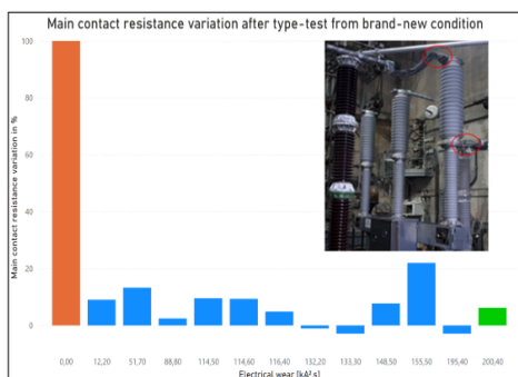
Figure 9 : Main contact resistance variation after type-test from brand new condition
