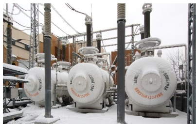
Fig.1 SFCL at substation in Moscow
