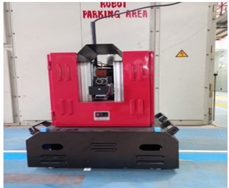
Figure-10: Robot images in switchgear room
