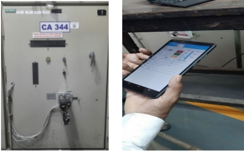
Figure-6: Motors mounted on the breaker panel & Mobile app
