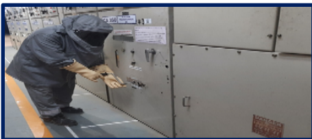
Figure-2: Operating person wearing Arc suit for carrying out rack in & rack out of breaker
