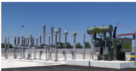
Ester insulated Current and Voltage Transformers 170kV installed on Italian Windfarm plant
