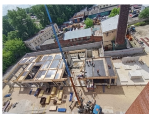
Main technological equipment building
