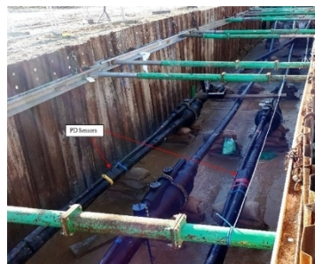
Figure 5: PD sensors close to the HV joints
