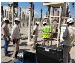
Figure 2. Training of company's staff on PD measuring equipment at a substation.
