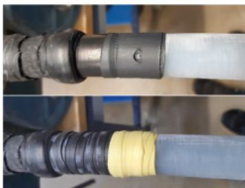
Continuous, Internal MV fault
