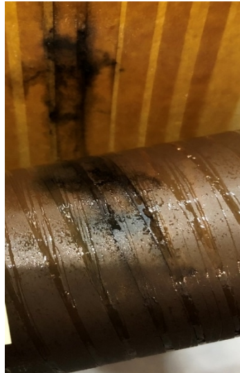
MIND cable insulation with carbonization damage caused by partial discharges.
