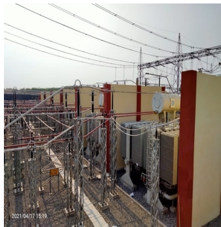
Figure 3 Multi level Substation
