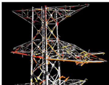
Fig.7 Example of rust extraction on the steel tower by AI
