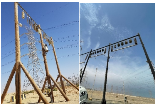
Fig (1) and (2) Al Fadhili KSA and Al Zour Kuwait Naturally Polluted Insulators Testing Stations.
