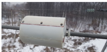
Fig. 2. Control device of the overhead line condition monitoring system installed on the conductor. This device measure conductor deviations and T parameter
