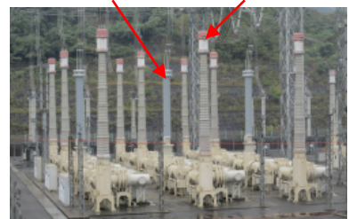
Overview of existing and replaced bushings
