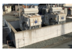
Fig. 16. Watertight wall around power equipment
