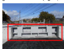
Fig. 11. Watertight gate at the substation entrance
