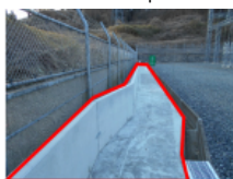
Fig. 10. L-shaped watertight wall around a substation
