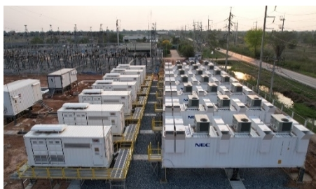
Figure II. Relocatable building (BESS in Thailand)
