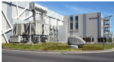
Figure-2 #2 HVDC Converter Station
