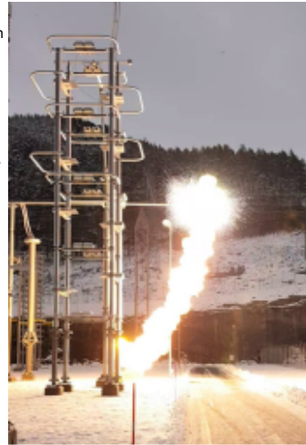
Field test 2 of a fault on the overhead DC line section of NordLink.
