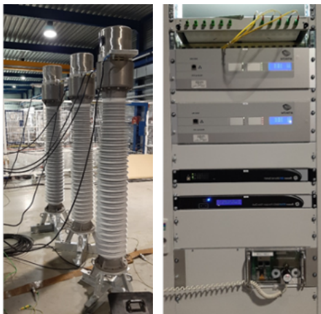
Fig. 1 OCT, merging units, metering unit, clock and switch
